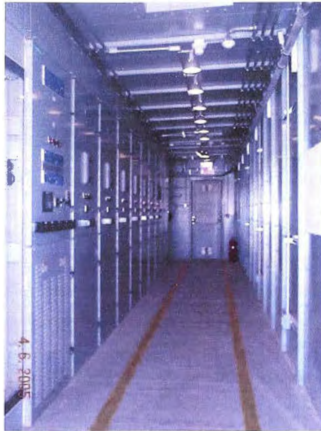
VISTA INTERIOR DE WALKING – SWITCHGEAR 13.8kV
