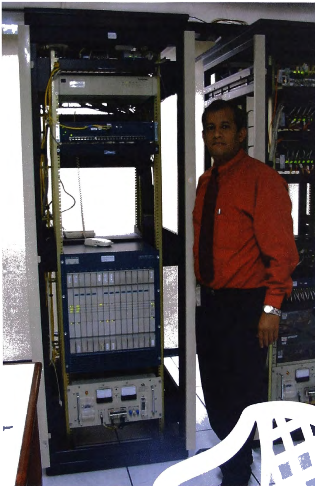
Figura A.8 - SWITCHING CISCO AS5300
