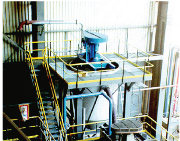
Flash Flote Cell in a Brazilian gold mine
