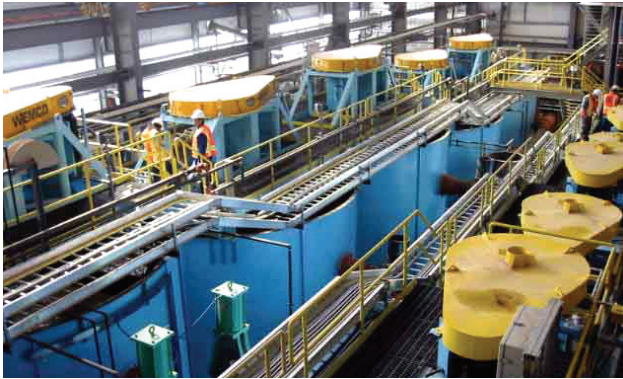
North American concentrator with 150 m 3 Wemco/Dorr Hybrid row. The Dorr-Oliver round tank cell includes many of the features developed for the world-leading Wemco® SmartCell® flotation machines.
