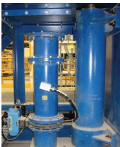
Air Control on Ambient Air Intake
