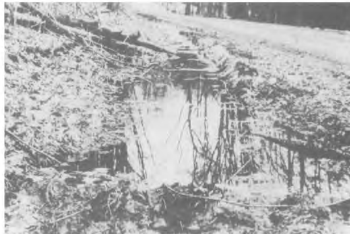
Figure B-4. High severity example of inadequate roadside drainage.
