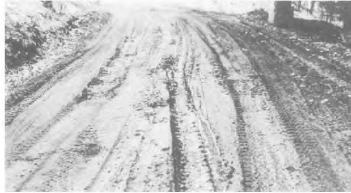
Figure B-2. High severity example of improper cross section.
