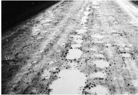
◀ Severe potholes covering most of road need additional gravel and regrading.
