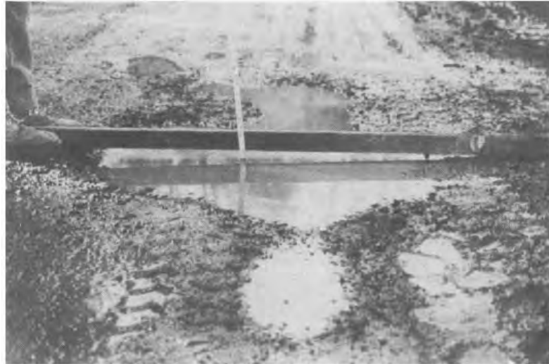
Figure B-10. High severity example of potholes.
