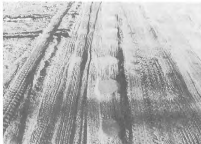
Figure B-6. Medium severity example of corrugations.
