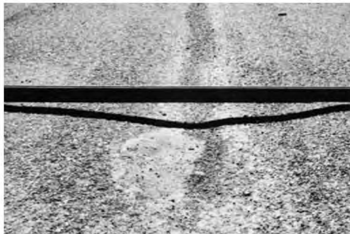
▲ Rut in wheel path needs regrading to eliminate ponding and prevent further road deterioration.
