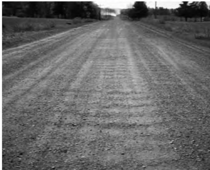
▼ Moderate washboarding in center of road.
