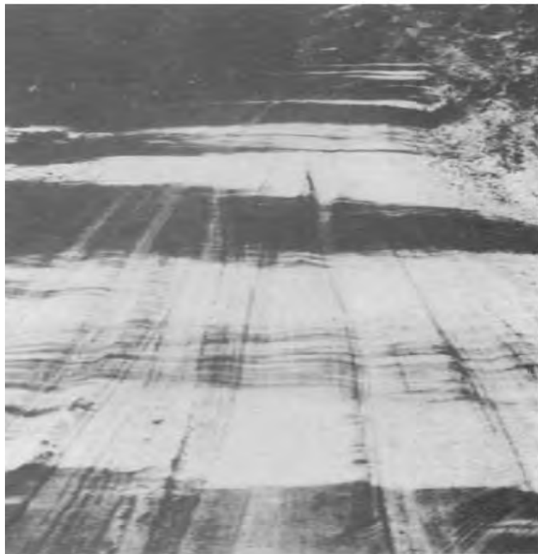
Figure B-12. Low severity example of ruts.
