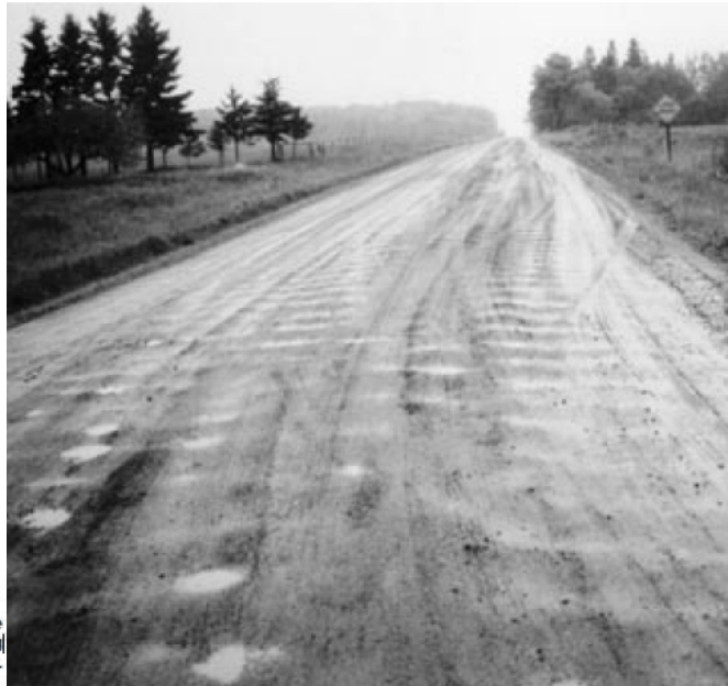
▶ Severe washboarding traps water.
