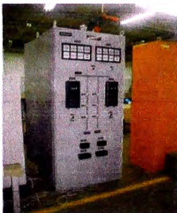
Figura 5.6. Tablero General MANELSA
