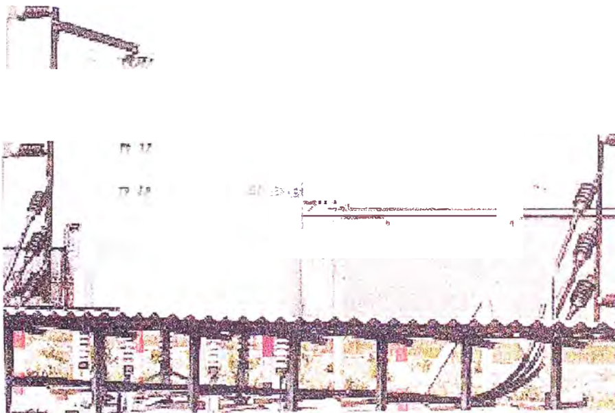
Fig. 5 Buffer reactor for E.A.F.
