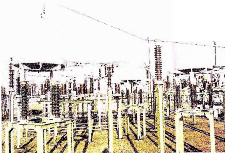
Fig. 3 Single phase series reactors
