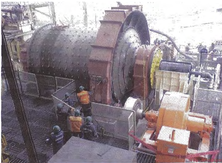
FIG 4.5 MOLINO FULLER INSTALADO
