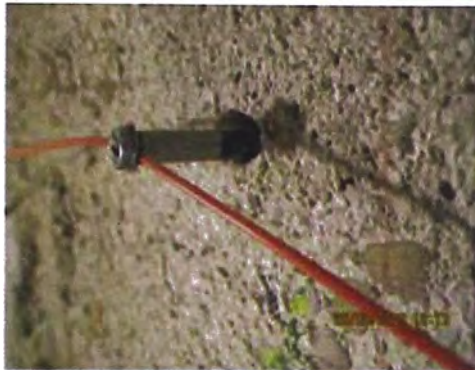
Anodos Titane Protection Cathodique (CPI)
