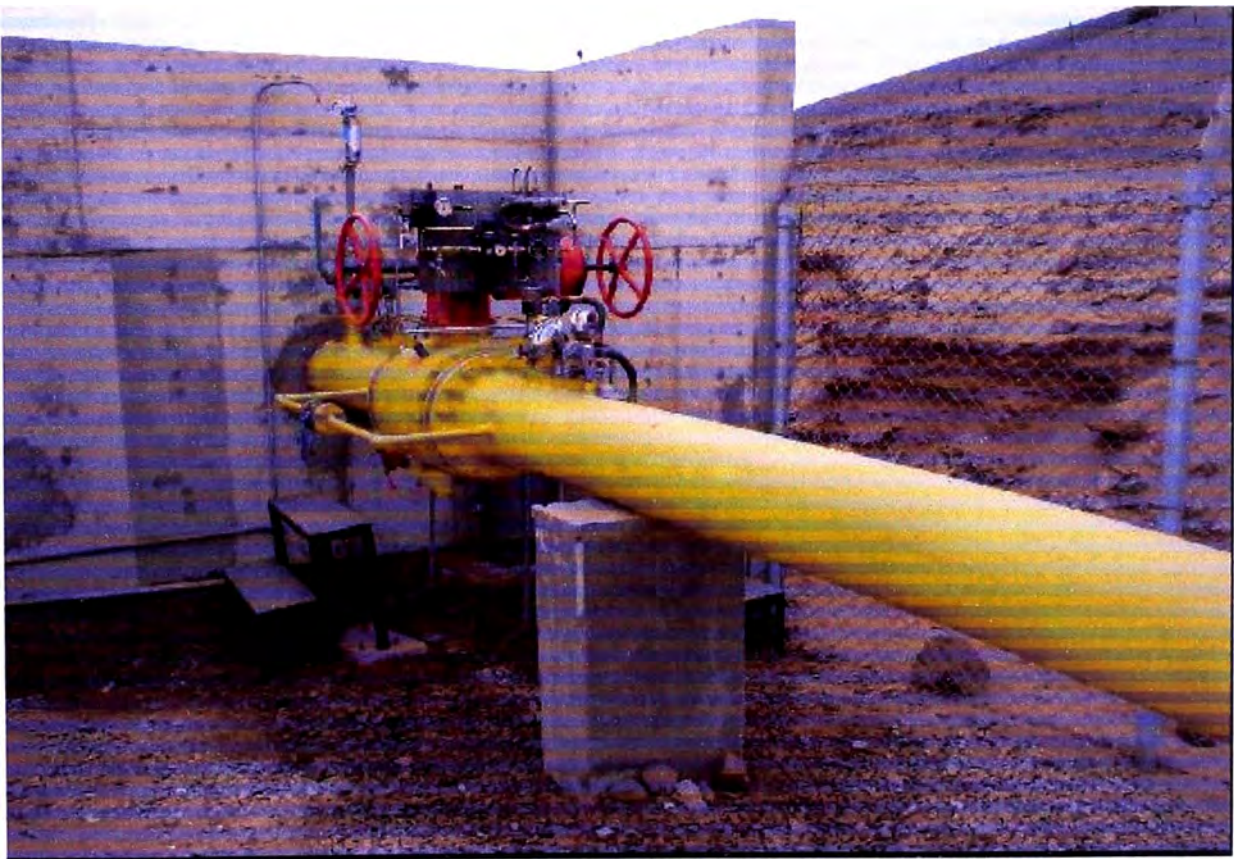
Figura 2.4: Suministro principal de gas natural
