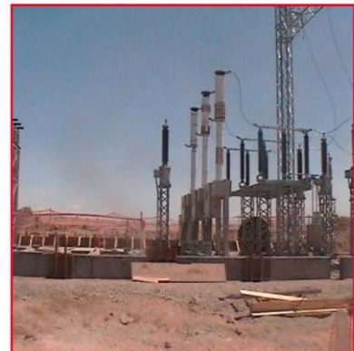
S.E. Central Panamericana Solar (23/138 kV)
