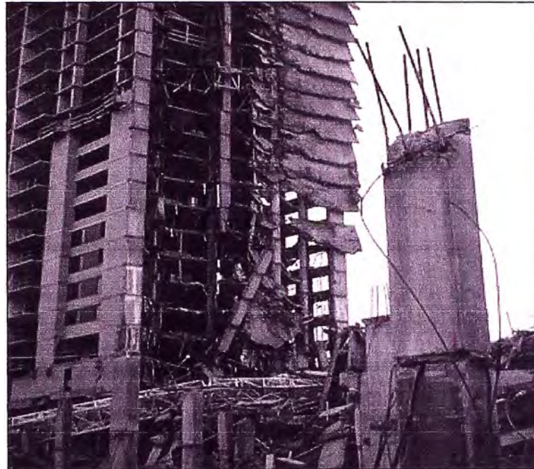
Figura 1.9 Skyline Towers Apartment. Colapso de pisos (13).
