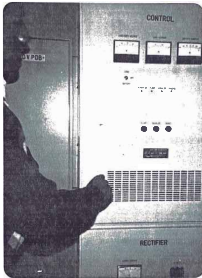
FIG. 5.12 PANEL DE CONTROL
