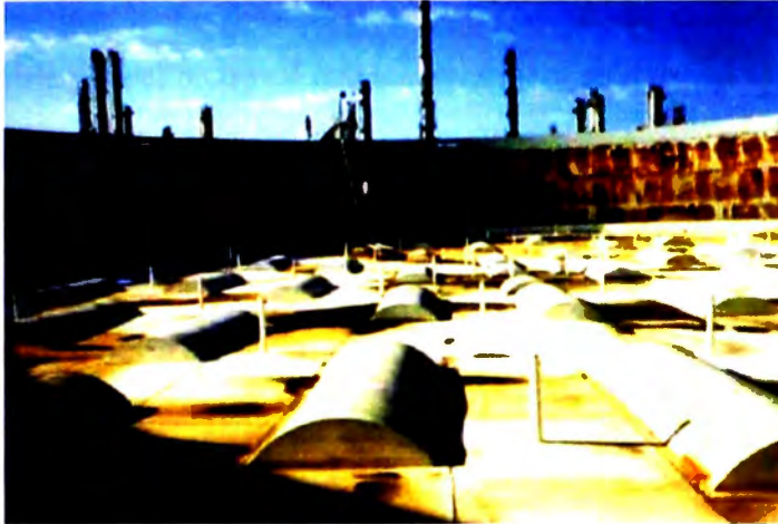
Fig 2.37 External Floating Roof of a Large Diameter Aboveground Storage Tanks
