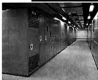
Central operation room (above) and high-voltage IGBT drive equipment (below)
